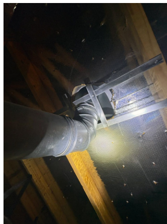
HVAC Gas Vent
